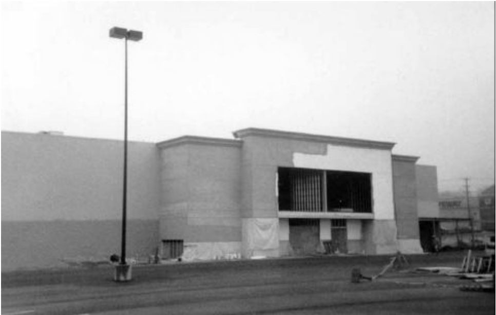
Sam's Club under construction in the redevelopment of Westview Shopping Center along Baltimore National Pike (Route 40 West).
